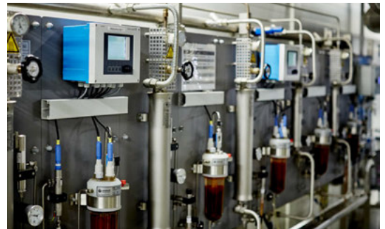
SWAS analytical panel for the water/steam cycle at the combined heat and power plant (CHP) Zwickau Süd
